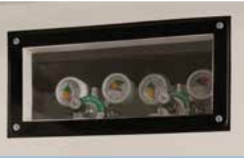
Oxygen manifold source and delivery system
